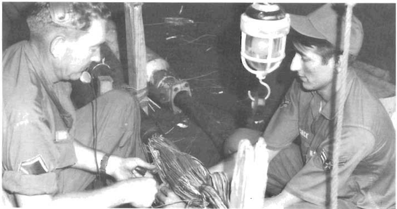
Damaged circuits required that AFCS technicians be constantly ready to provide repair services to insure continued operation of important communications facilities.
