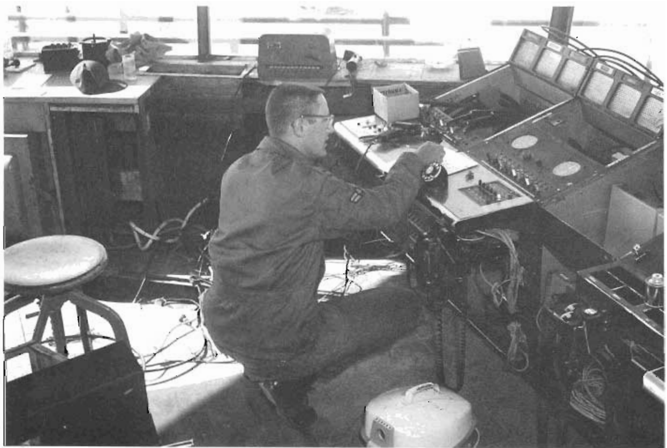
A control tower is just as much an integral part of the Air Force as an airplane. Here, an AFCS technician rewires the control tower as part of the continual rehabilitation, modification, and maintenance efforts to ensure adequate support of aircraft.
