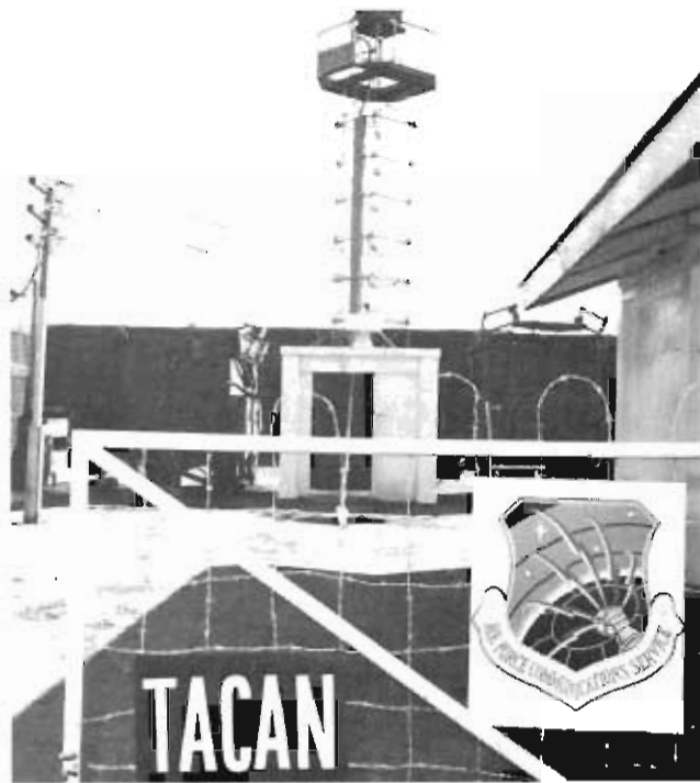
AFCS provided a wide variety of communication equipment to support the Air Force effort in Southeast Asia. This tactical air navigation facility at Pleiku AB, South Vietnam, provided en route and terminal navigation assistance to aircraft.
