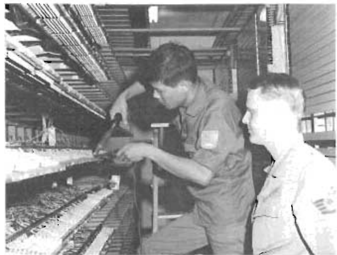
A vital preliminary to turning over dial central offices at Vietnamese bases to the Republic of Vietnam Air Force was the training of Vietnamese in maintenance procedures. Here, an on-the-job trainee soldiers a connection among the maze of wires making up the dial central office at Binh Thuy AB, South Vietnam, as a member of the 1880th Communications Squadron observes.
