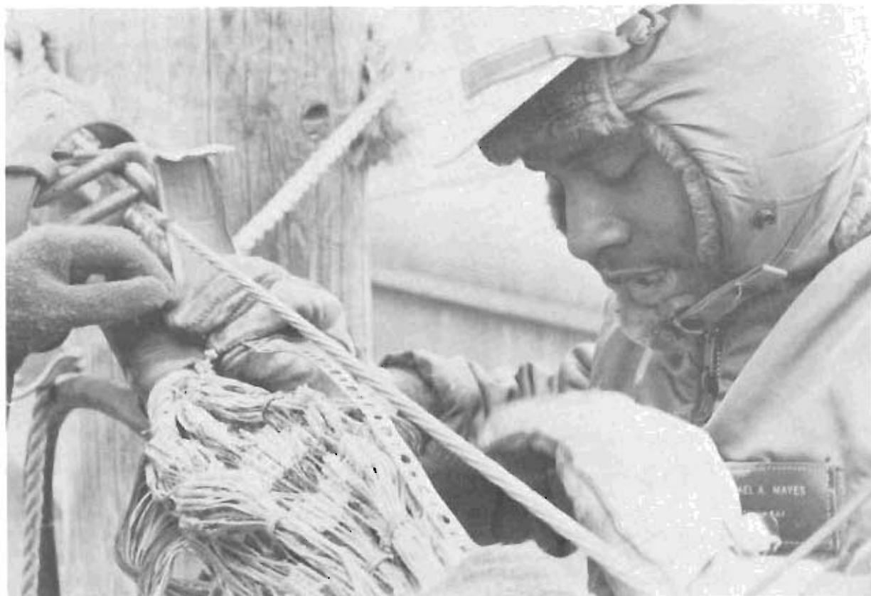
In subfreezing temperatures, a member of the 1839th Engineering Installation Group fastens a 100-pair bridge to a 400-pair cable during a cable expansion project at Incirlik AB, Turkey.
