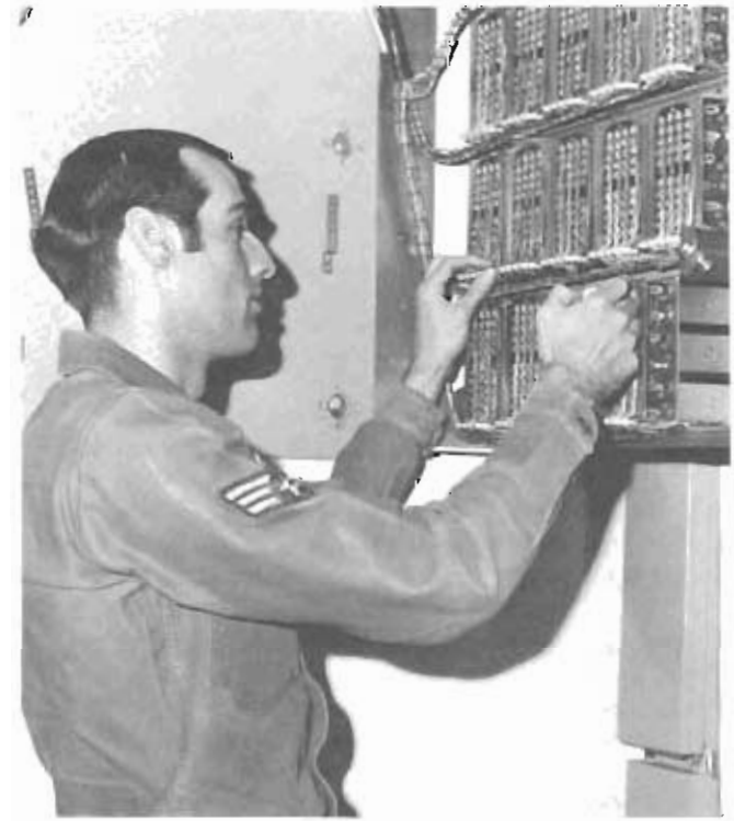
An AFCS airman checks the relays used in a telephone key system. A relay panel such as this one can carry as many as 50 dial or 20 direct lines.
