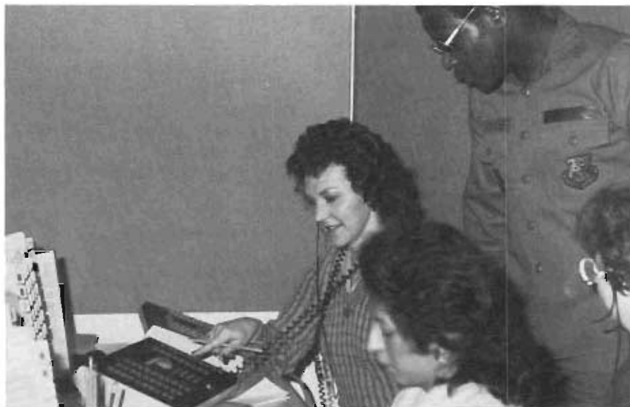
CMSgt Burt Skinner, right, the superintendent of operations for the 1923d Communications Group, is shown some of the new computerized telephone operator consoles that replaced the old patch cord type switchboard at Kelly AFB, Texas. The new equipment was approximately one-tenth the size of the old equipment, but had many more capabilities, such as call transfer and three-way calling.
