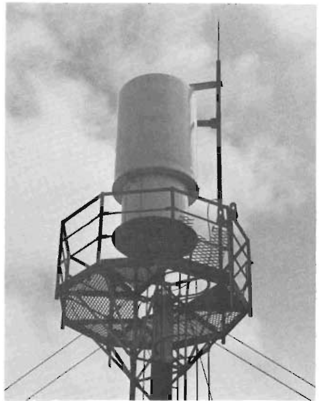
In March 1985, AFCC installed a prototype of a TACAN antenna (AN/GRA-121) with a heated radome at Shemye AFB, Alaska. The heat made the antenna, used for enroute and terminal service, invulnerable to blowing snow and ice buildup.
