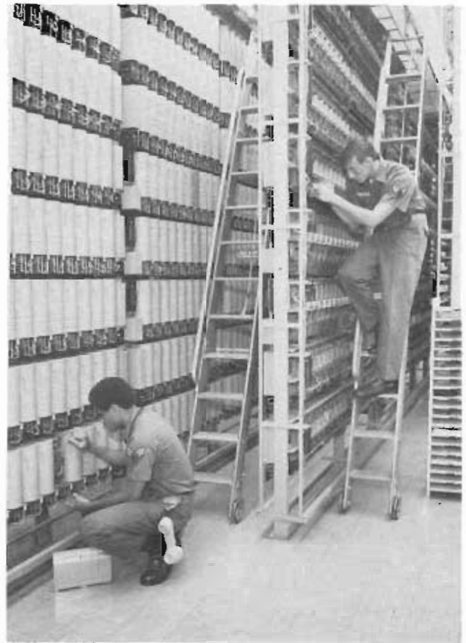
AFCC maintenance workers check wiring connections in the old telephone central office at Kelly AFB, Texas.
