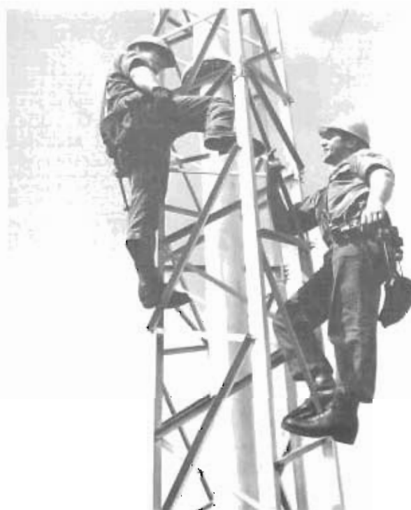
Air National Guard technicians, during their two-week training stint with AFCS, work on an antenna being installed on the island of Antigua in support of a NASA space flight. AFCS personnel have helped maintain the communications link with the astronauts on every manned space flight.
