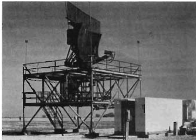
An AN/GPN-20 radar surveillance antenna with the fixed site/false target antenna mounted on top of the radar antenna.
