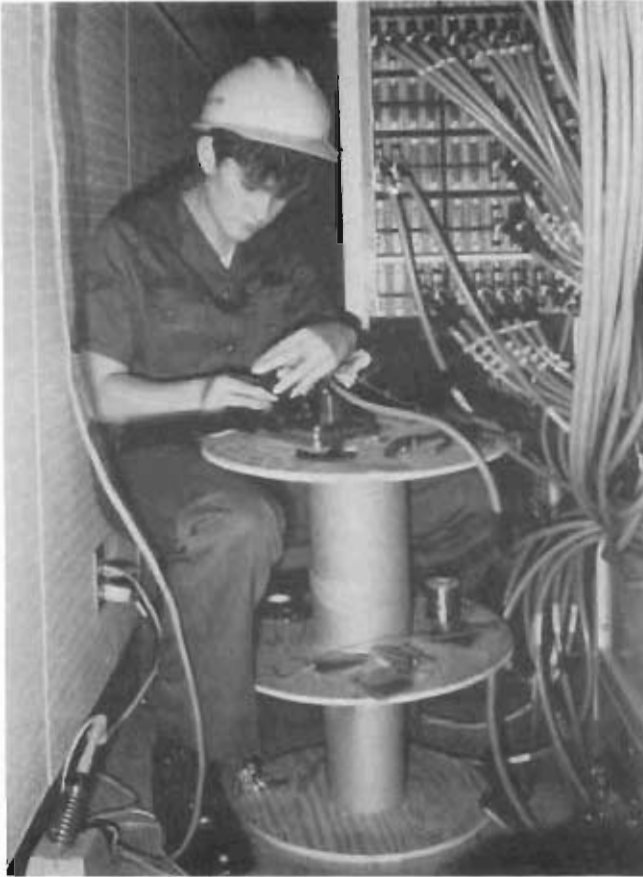
A1C Sharnee Riley, radio team member, 1837th Engineering Installation Squadron, uses an Amphanol "Amp-Champ" crimper to terminate a connector on one of the multitude of 25-pair cables installed at the control site as part of the Scope Signal III installation at Clark AB, Philippines. Scope Signal III is the program to modernize Giant Talk, the Strategic Air Command's world-wide command and control network. The station at Clark was the first Air Force-installed station to come on line.
