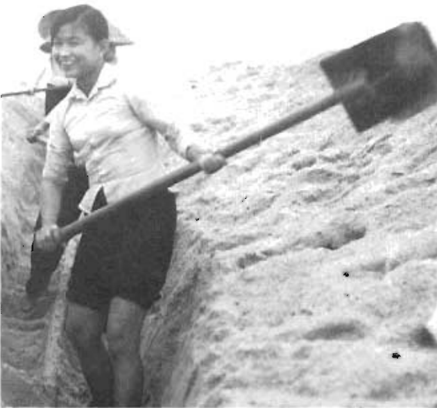
Vietnamese girls aided in the effort to complete the underwater communications system by digging trenches for the cable on the beaches.
