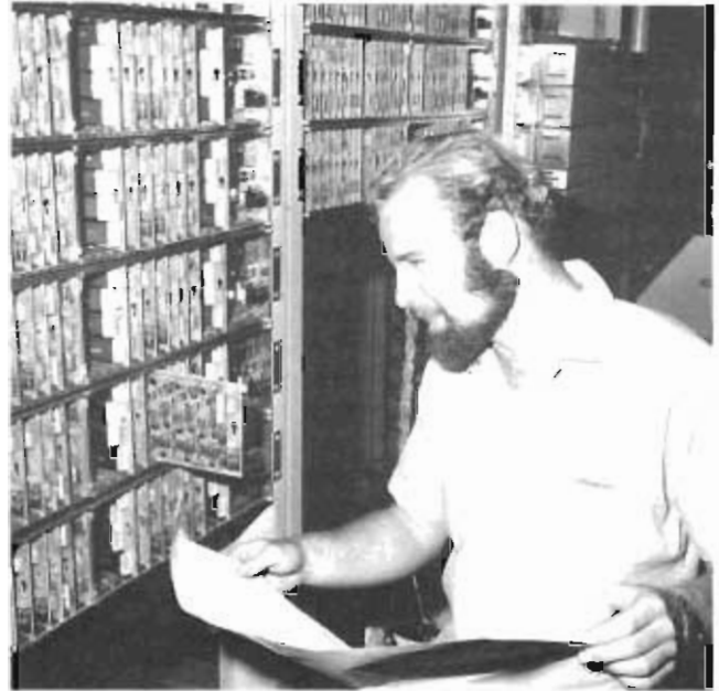
Utilizing civilians to augment military personnel in Southeast Asia relieved some of the manning problems. Here, a civilian technician inspects a tandem switch at Pleiku AB, South Vietnam, which will give the base and the surrounding area direct, long-distance dialing capability.
