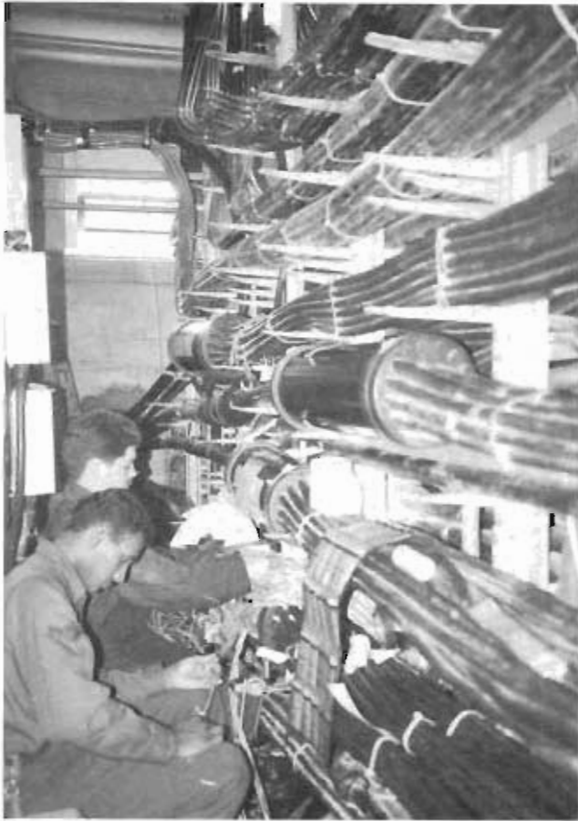
Sgt Charles Budd and Amn Nalim Ali of the 485th Engineering Installation Group splice a 3,000-pair cable in a cable vault at Wright-Patterson AFB, Ohio.
