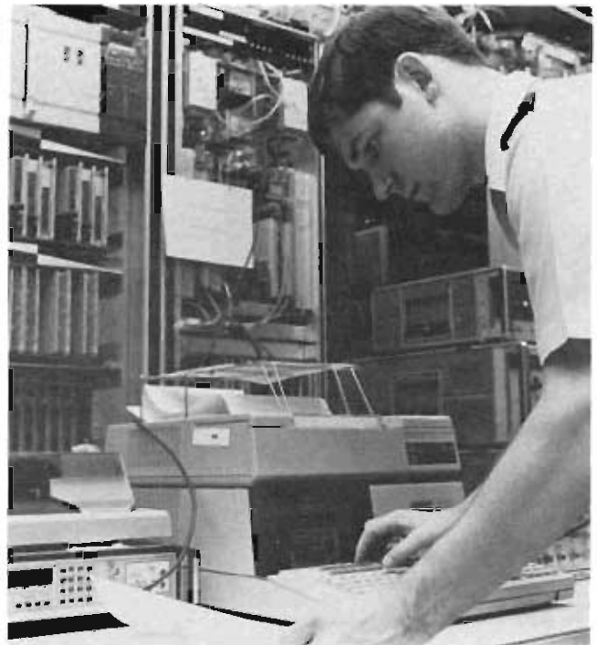
2LT Norman Howard, 1842d Electronics Engineering Group, verifies automated procedures on the prototype digital microwave radio system. This installation supports the Japan Reconfiguration and Digitization program. These radios are now being installed at various sites in Japan and the automated tests are used to verify system performance and accomplish test and acceptance in the field.
