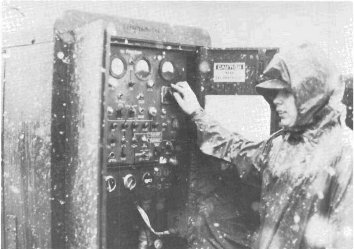
An MB-Teen series mobile generator is used to power information systems equipment during deployments or contingencies.
