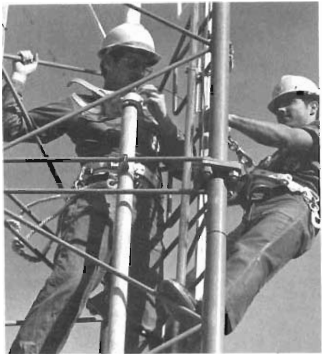
Members of the 1923d Communications Installation Group, Kelly AFB, Texas, install conduit on the glide slope antenna tower. The tower is part of a new electronic system (the GPN-29 solid state instrument landing system) that guides aircraft to the primary landing runway at Holloman AFB, New Mexico.
