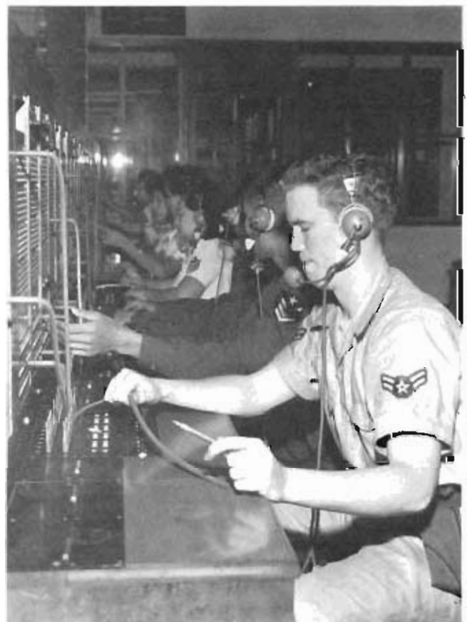
The switchboard at Don Muang AB, Thailand, manned by AFCS and Royal Thai Air Force personnel, provided telephone support to forces early in the sixties.
