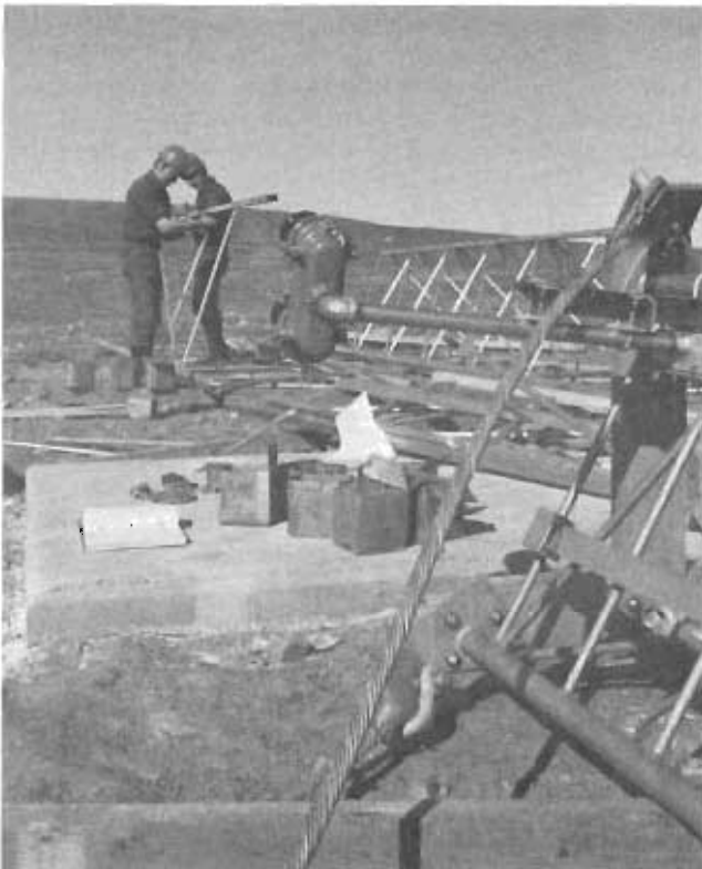
SrA Sid Trekel and A1C Mike Trevizo of the 485th Engineering Installation Group complete the boom section of a heavyweight rotatable log antenna on North Mountain, near Thule AB, Greenland.
