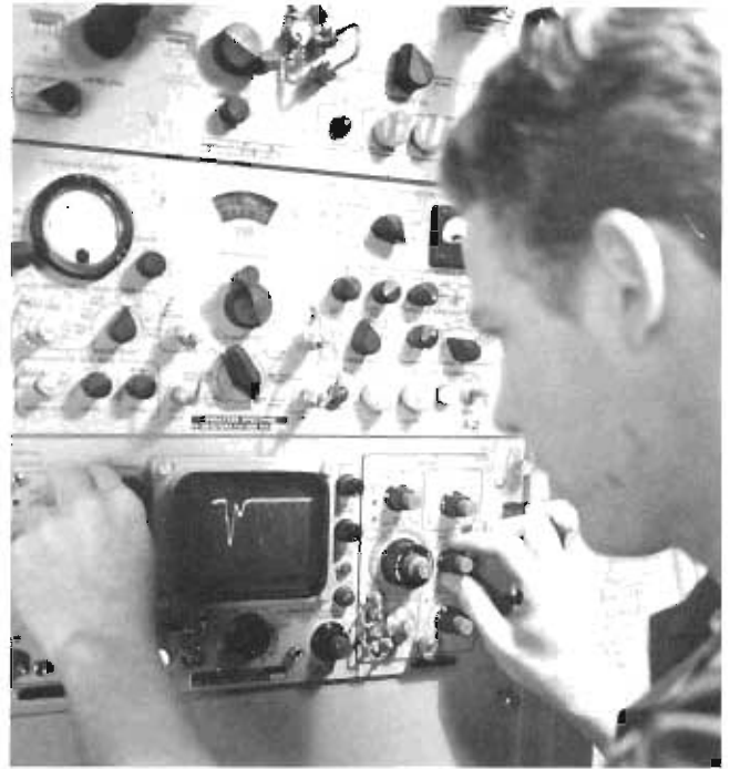
An AFCC technician inspects equipment at a Tactical Air Navigation site to ensure it is getting the proper amount of power.
