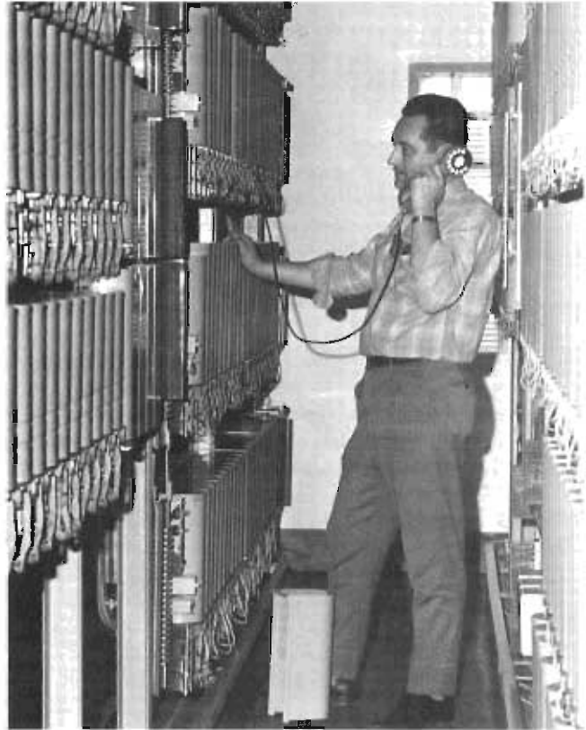
There's more to using the phone than just dialing a number. A constant check on telephone circuitry is necessary to ensure that phone service is kept reliable. Here, a telephone repairman checks a trouble call to keep the AUTOVON network running smoothly.
