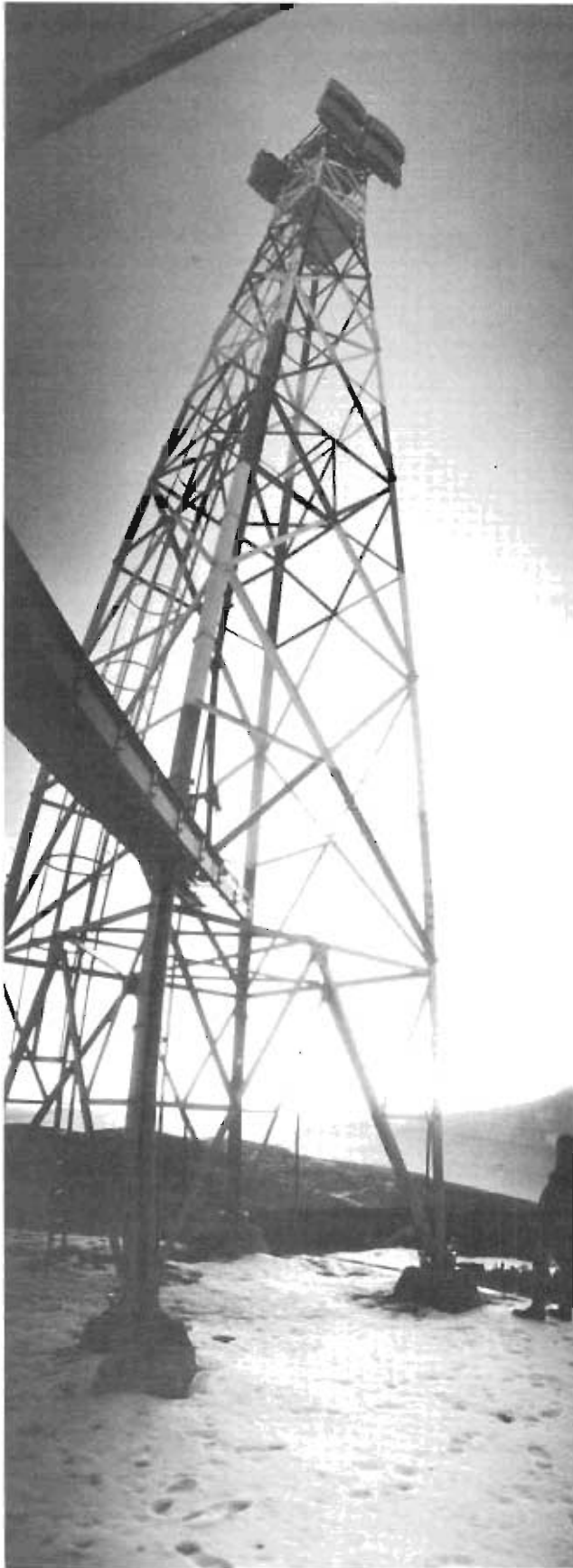
An antenna tower on Mt Paganella, Italy.
