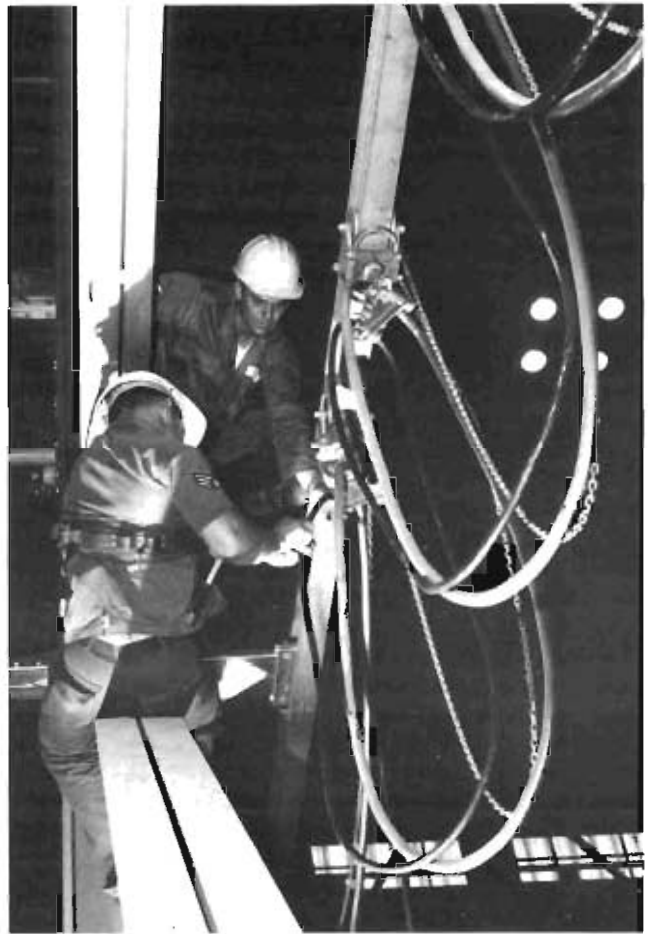
High riggers from the Ground Electronics, Engineering, and Installation Agency install cables on a mobile service tower at Cape Kennedy AFS, Florida, prior to a missile launch.
