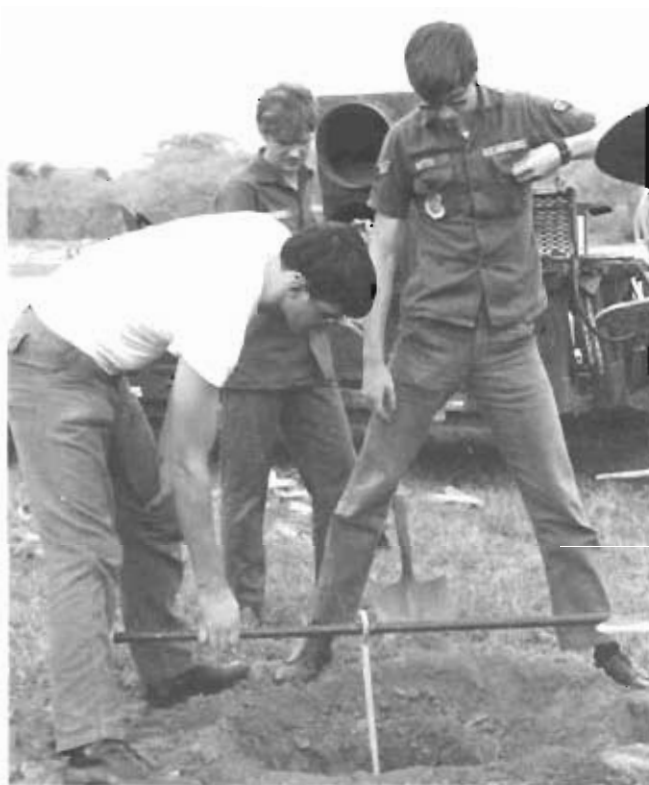
Three AFCS airmen install a ground rod for a mobile control tower.
