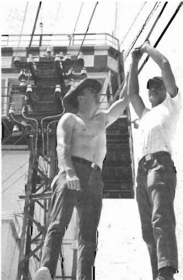
Two AFCS outside maintenance men work on telephone lines below the control tower at Tan Son Nhut AB, South Vietnam.
