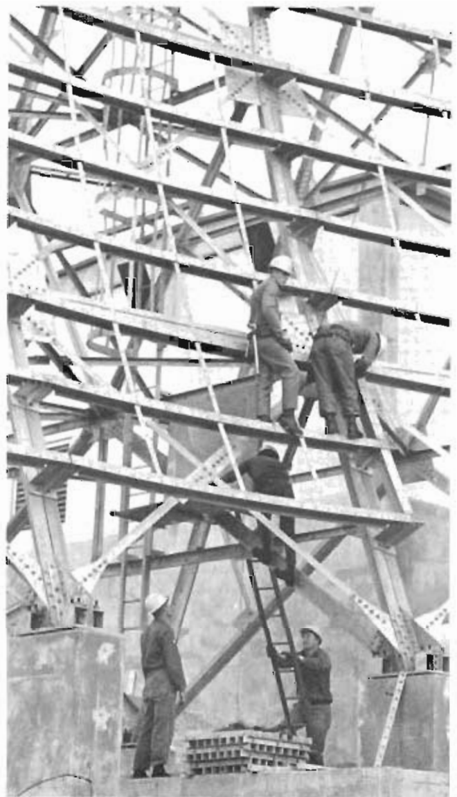
GEEIA member construct a microwave antenna at Izmir, Turkey, for use by AFCS.
