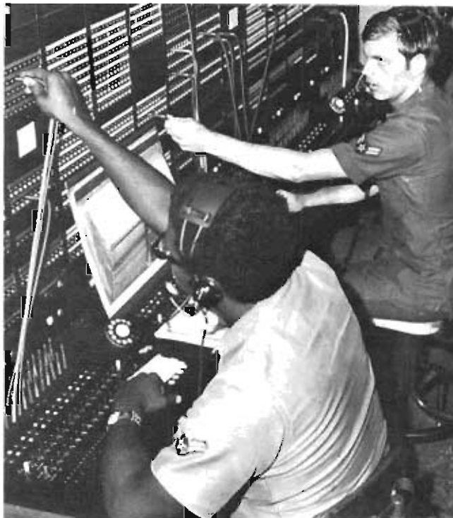
Switchboards such as the one pictured were operated by AFCC to provide efficient and accurate telephone services to the Air Force.
