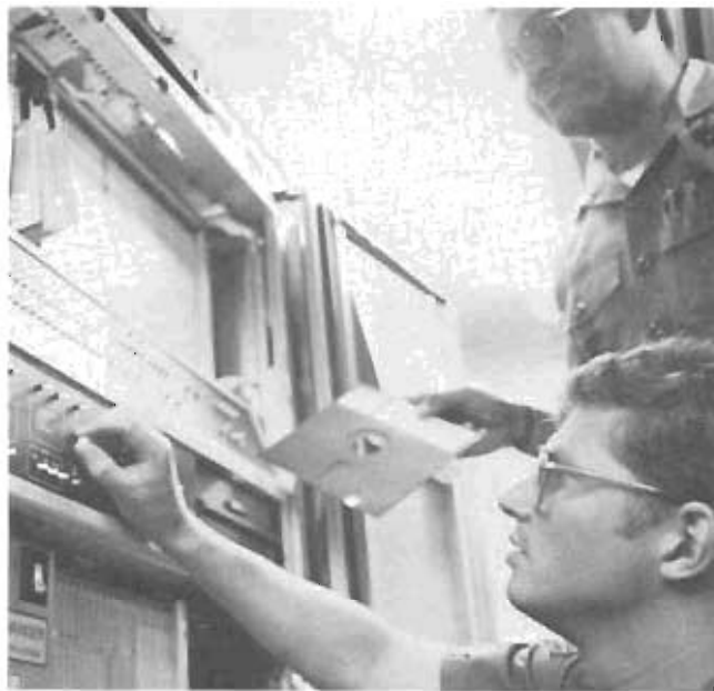
SrA Larry Psenick, 1956th Communications Group, Yokota AB, Japan, sets address switches on a disk controller while TSgt Charles Ross, 1982d Communications Squadron, Kunsan AB, Korea, stands by with a boot floppy disk. The two were testing part of the data processing Tactical Shelter System, a transportable base data processing system designed to provide automated base level information systems support under wartime or contingency operations.
