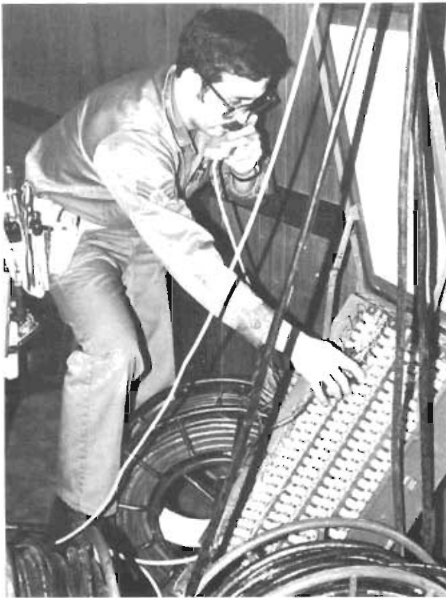
An outside plant technician with the 2063d Communications Squadron, checks connections on some of the thousands of feet of telephone cable installed for news media and the State Department when the returnees were brought to the USAF hospital at Wiesbaden AB, Germany.
