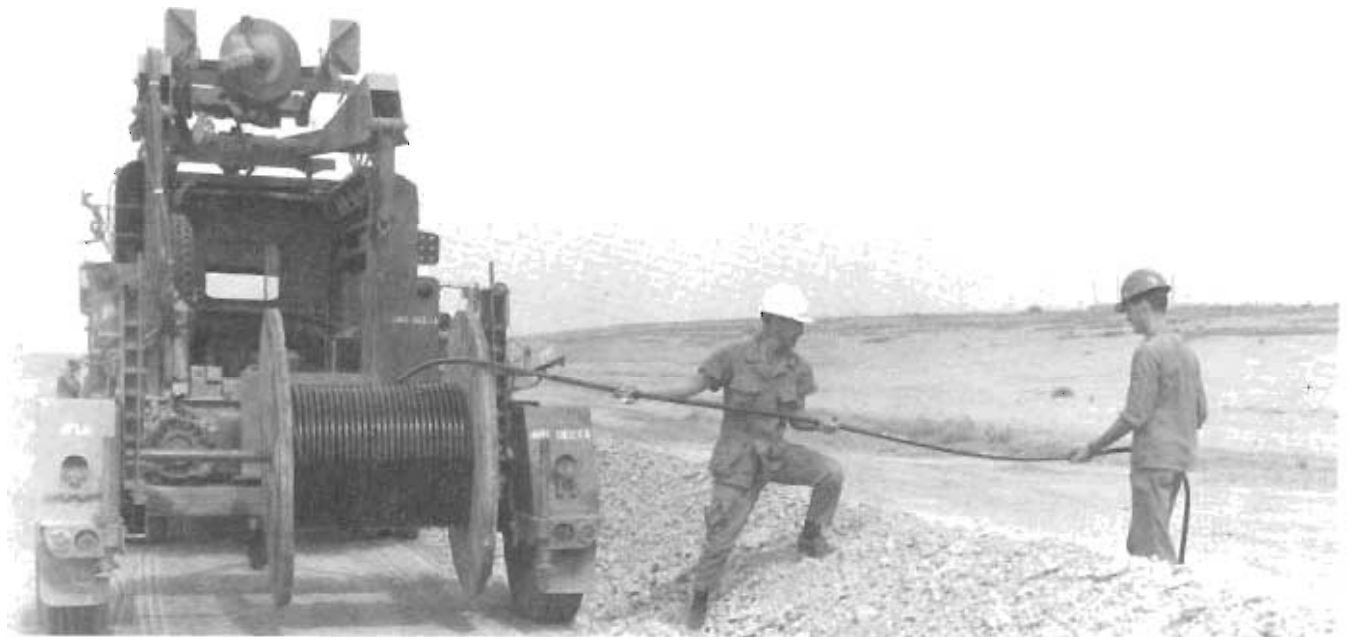
Members of the 1B77th Communications Squadron at Bien Hoa AB, South Vietnam, feed telephone cable into a ditch.
