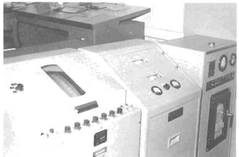
This portion of the AN/TMQ-11 indicates the temperature and humidity information it receives from the remote transmitter located on the airfield.
