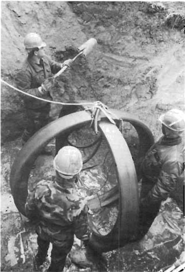
A1C Charles Atwood, with shovel, SrA Floyd Homer, and Sgt Christopher Fowler, 1827th Electronics Installation Squadron, prepare the survivable low frequency communications systems antenna.
