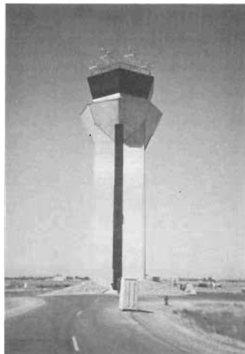
On 20 September 1985, the Army Corps of Engineers transferred the new control tower at Mather AFB, California, shown here under construction, to the base civil engineers.
