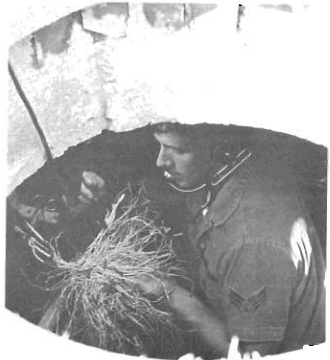
A cable splicer with the 1974th Communications Group works in a manhole at Scott AFB, Illinois.
