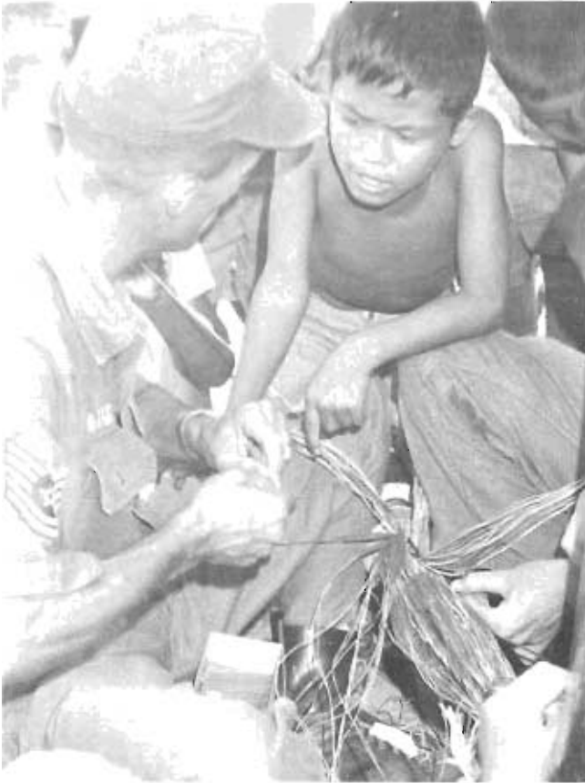
Local children observe a communications technician splice cable at Don Muang AB, Thailand.
