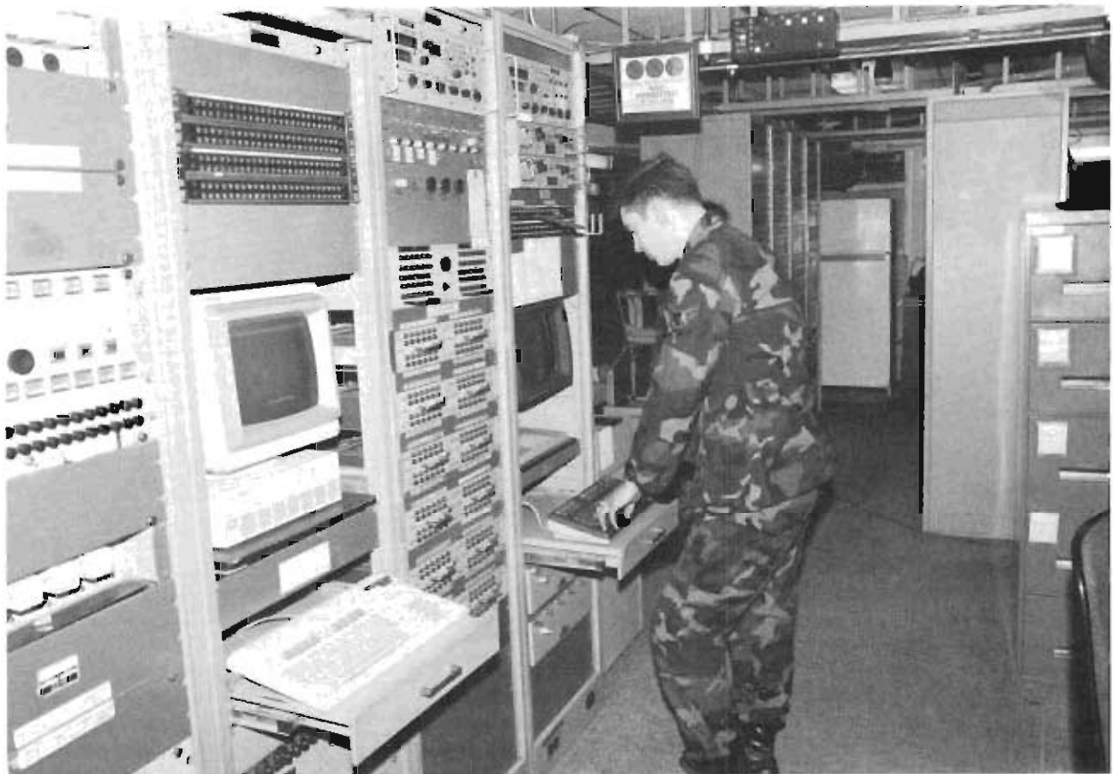
A1C Mark Williams checks the status of Digital European Backbone remote unmanned sites using transmission monitoring and control equipment.
