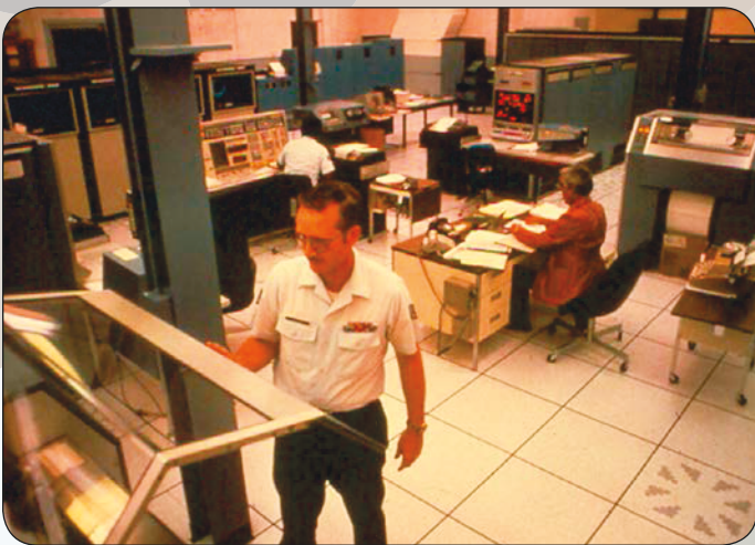
Interior view of an AUTODIN automatic switching center.
