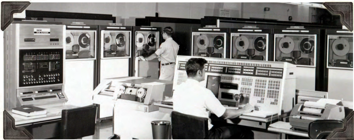
Interior view of the McClellan AFB AUTODIN Switching Center.
