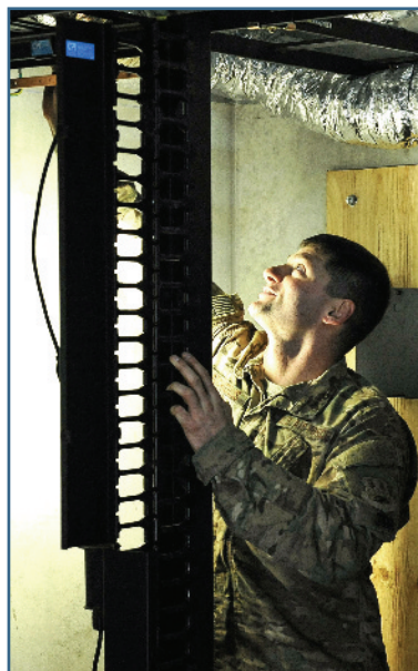
SSgt. Patrick Little, cyber transport supervisor, removes a back-up power supply from a darkened storage area at Bagram Air Field. (AF photos by TSgt Nicholas Rau)
