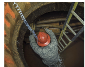
Airman Clayton Perry, 633rd CS, cable and antenna systems technician, works in a manhole. The Operations Flight maintains 90 miles of copper cabling, 600 manholes, 22,000 computer systems, 17,000 phones and 18,000 user accounts.
