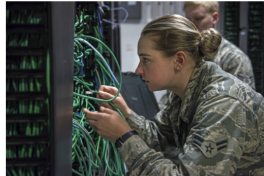
A1C Victoria Nowak, 633rd CS cyber transport technician, patches a computer to the network to give it connectivity at Joint Base Langley-Eustis.
